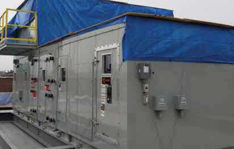
Left: A standard-size energy recovery unit barely fit through the double doors at Mariucci Arena. // Middle: At Mariucci Arena, each locker has exhaust fans to dry out equipment. // Right: Rooftop Air Handling Unit at the Mechanical Engineering Building
